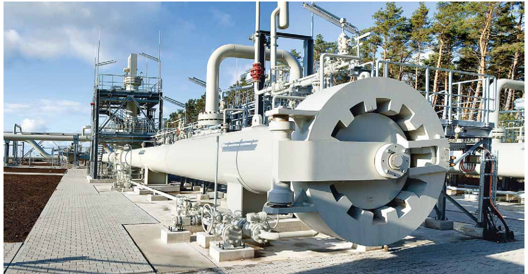
Above, a Pipeline Inspection Gauge (PIG) trap, houses the PIGs that have traveled through the pipeline from Russia.
